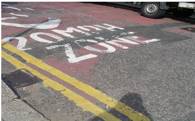
Deteriorating surface markings on 20mph signs should be repainted
